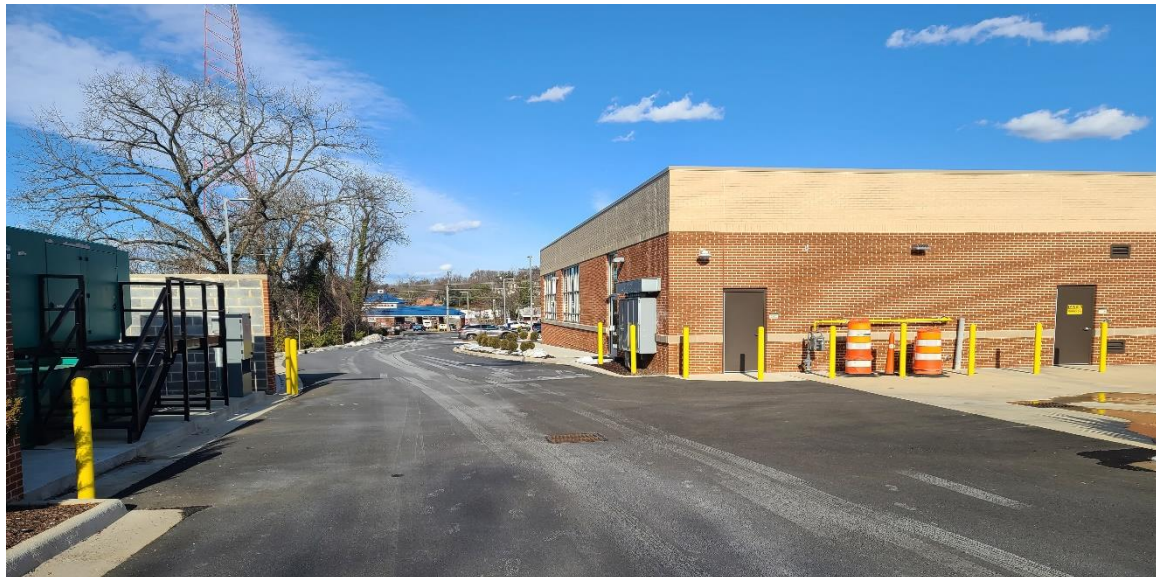
Charlie Delta Corner with gas shut off behind the construction barrels, electrical panel on side delta, and generator to the left.
